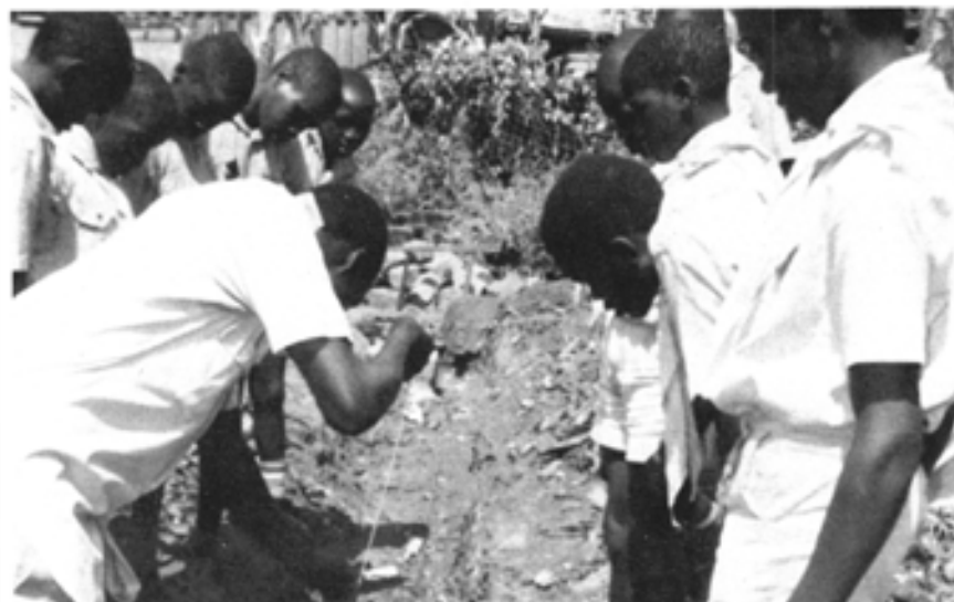
A technical expert shows Bwaise Scouts how to level the foundation before laying handmade bricks to build a chicken house in Kampala District, Uganda. The poultry project, sponsored by the Blue Water Region, Ont., gave groups like the 4th Goderich some fun, too, says Mary Anne Rowlands, field executive. During the promotional meeting, live chickens paid a visit and Goderich Beavers decorated the walls with their posters of chickens and chicken farming. The Egg Marketing Board let the group use "Let's Get Cracking!" materials for fundraising and, each time an egg was cracked in a member's home during March, 10 cents was put aside for the poultry project. Mary Ann says the 4th Goderich raised almost $800 for Uganda.
